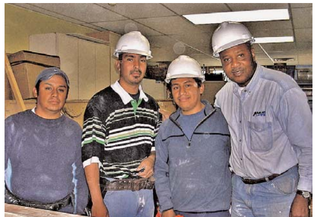
Harold Hardy, far right, of Hardy Property Services, LLC and his crew are installing windows in the art room, science room and supervisor’s work room to let in more light and allow for better supervision.
