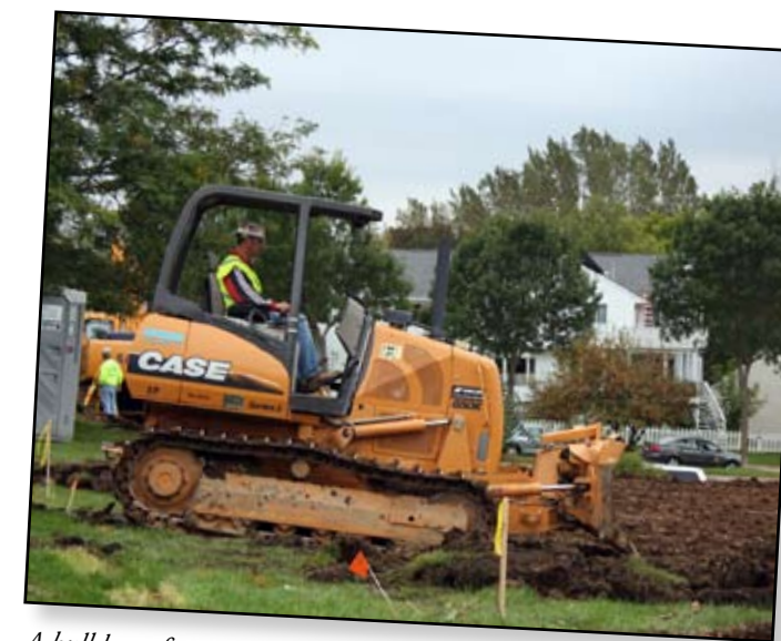
A bulldozer from Homburg Contractors Inc. works on the expansion of the parking lot at the administration building.
